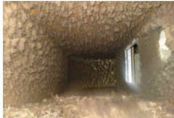
Excessive Grease Fouling
